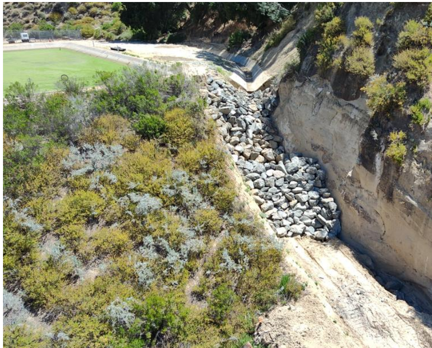
Figure 31: Drainage Channel Blowout and Stabilization of Embankment
