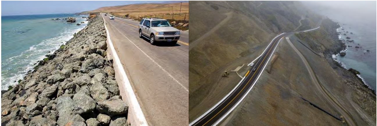
Figure 5-40 Vulnerable Portions of Highway 1 and Realignment near Piedras Blancas
