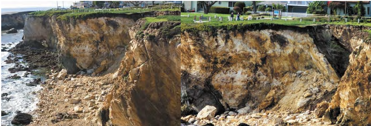
Figure 5-35 Bluff Erosion and Overlying Development at Dinosaur Caves Park in Pismo Beach, January 2010
