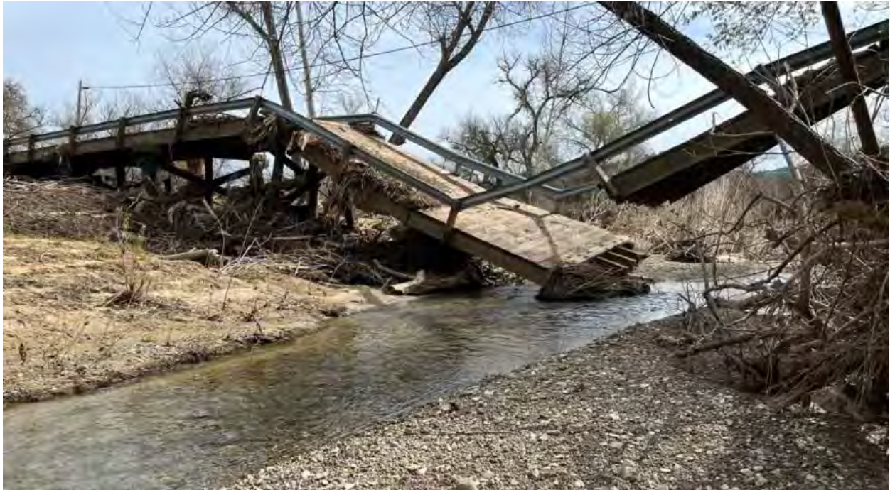
Figure 5-84 2023 Flooding Damage– Huasna Townsite Road
