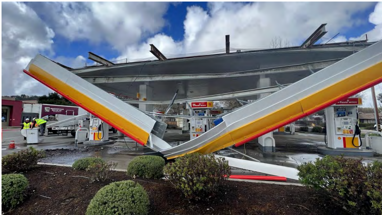
Figure B-3 High Wind Damage to Gas Station in Atascadero
