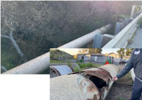
2 Whale Rock: The Whale Rock Pipeline is aging, but has benefited from targeted infrastructure upgrades, and replacing older segments with modern materials to extend service life.
