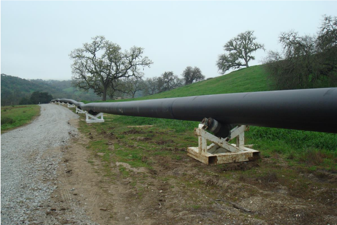
Figure 3. Example of a Pipeline Roller Stand
