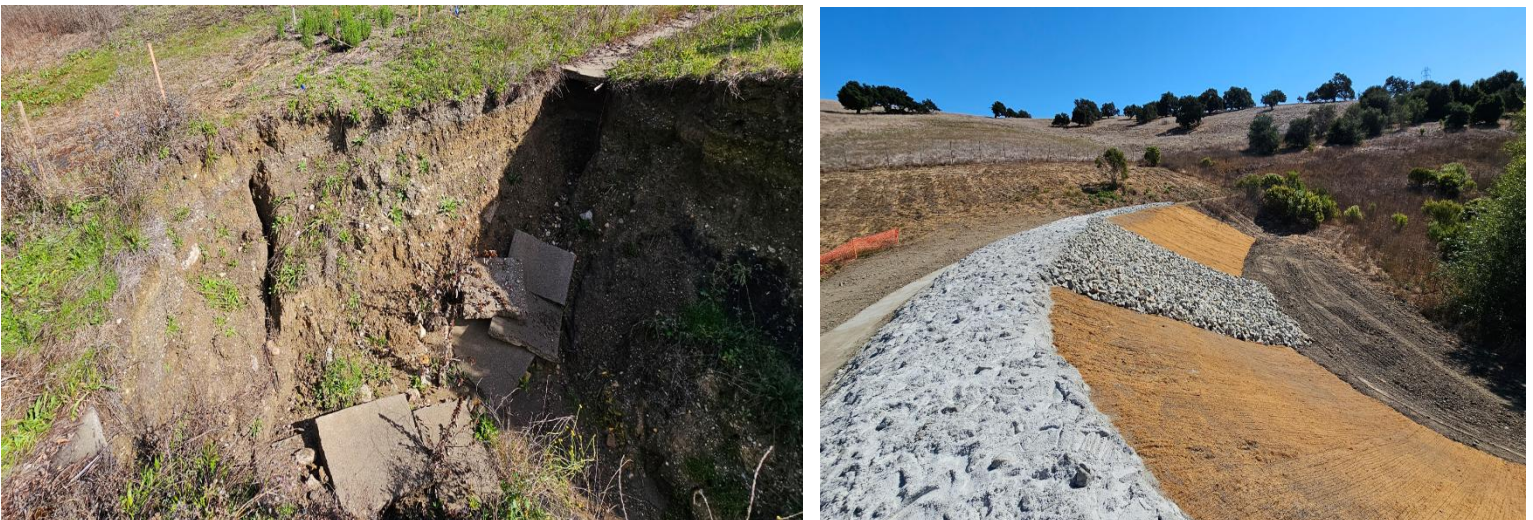
Figure 24: Perimeter Channel Breach Before Repairs vs Perimeter Channel After Repaired
