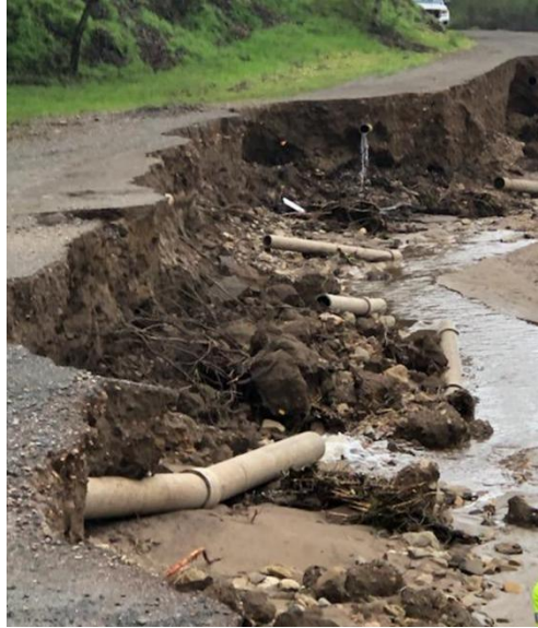
Figure 28: Lopez Lake Treated Effluent Line Break
