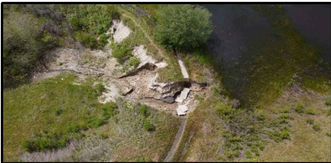
Figure 22: Perimeter Channel Breach on North Side of Terminal Reservoir
