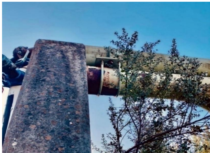
Figure 8: Sewer Force Main Wear or Corrosion
