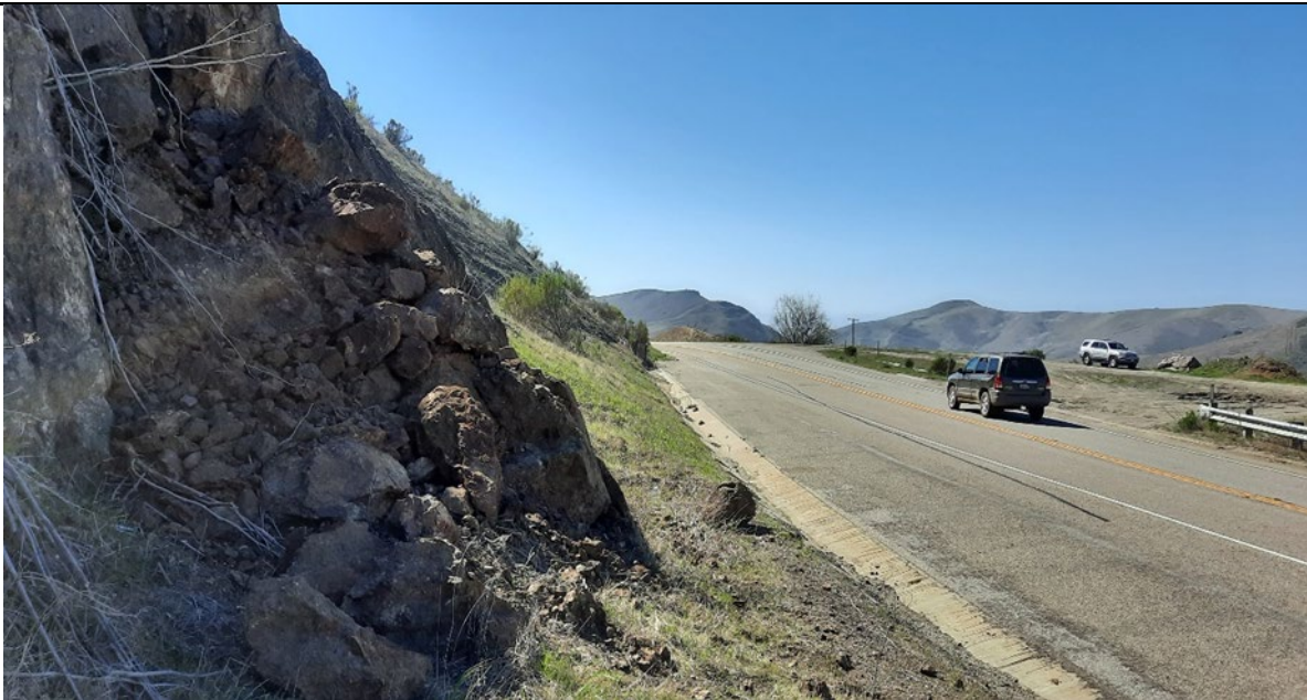
Figure 4: Landslide on Old Creek Road
